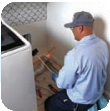
Dryer Vent Cleaning
